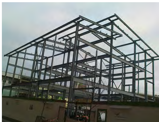
A building under construction. You can see the framework made of steel.
