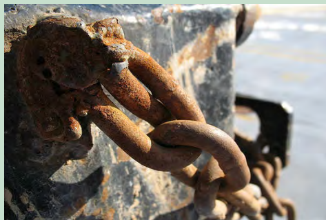
A rusted chain.
