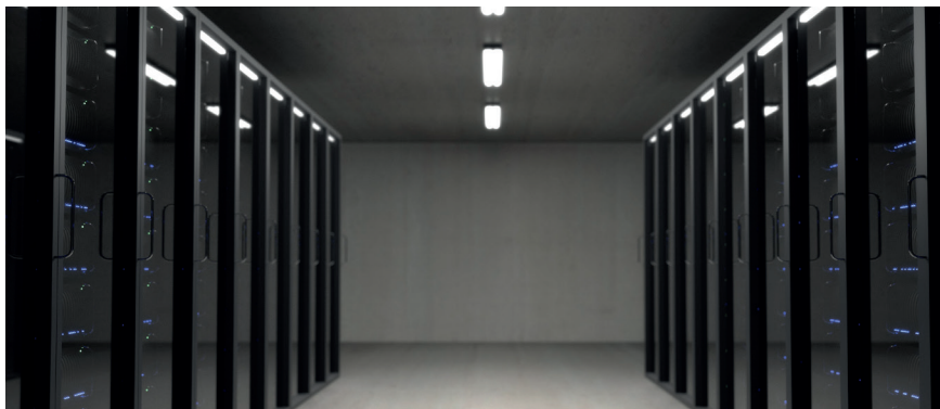
Figure 6.1: Data centres can contain hundreds of powerful servers
