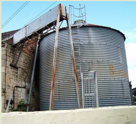
A tank made from corrugated iron. 2
