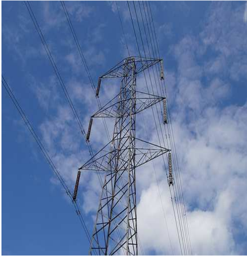
A pylon is a frame structure that supports electricity lines. 3
