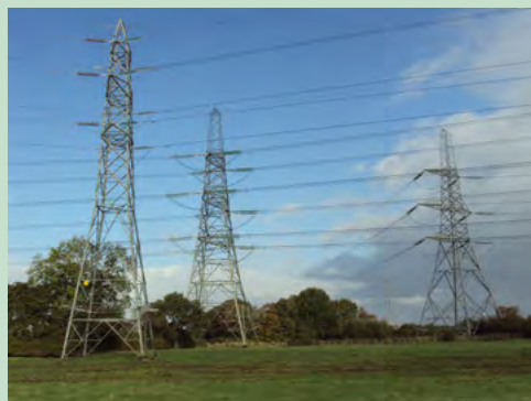
These electrical wires carried by pylons are made of metal.
