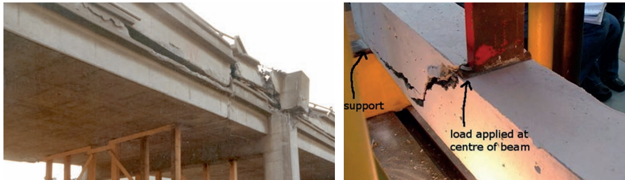
Figure 5.7 Shear failure in a concrete column and a beam
