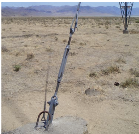
Figure 3.17a Cable stabilising a tower
