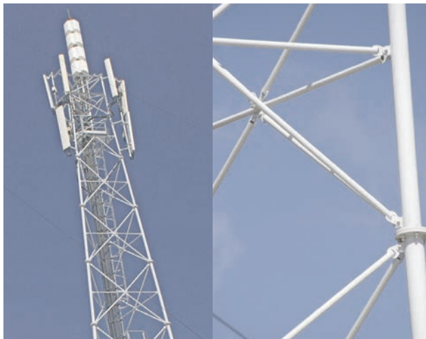
Figure 3.20a The steel columns of this cell phone tower are heavier than all the other members
