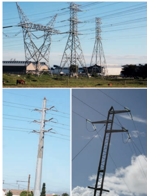
Figure 2: Different types of electricity pylons
