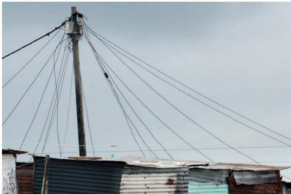
Figure 5: An informal community with an electrical supply. Notice the control boxes at the top of the poles. They control how much electricity each household uses and have a built-in safety mechanism for when there is a short circuit.
