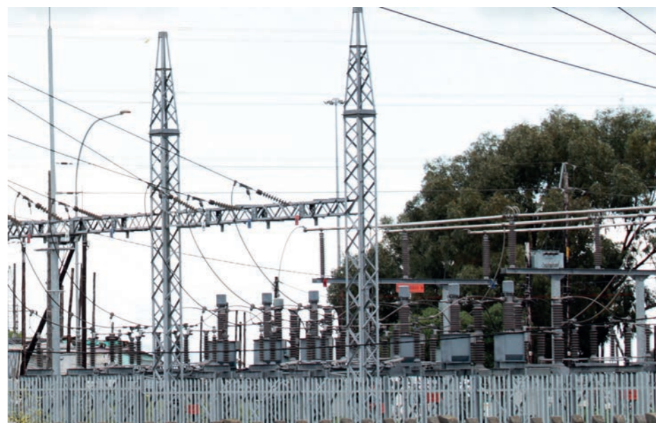
Figure 8: An electrical substation. These are often targeted by electricity thieves.
