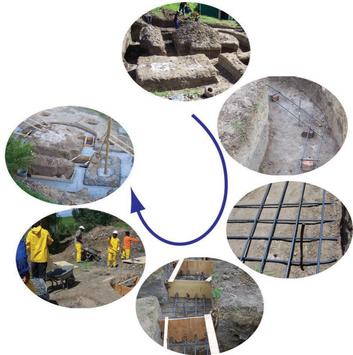
Figure 18: Steel reinforcement is used to strengthen the concrete foundations of a new house.
