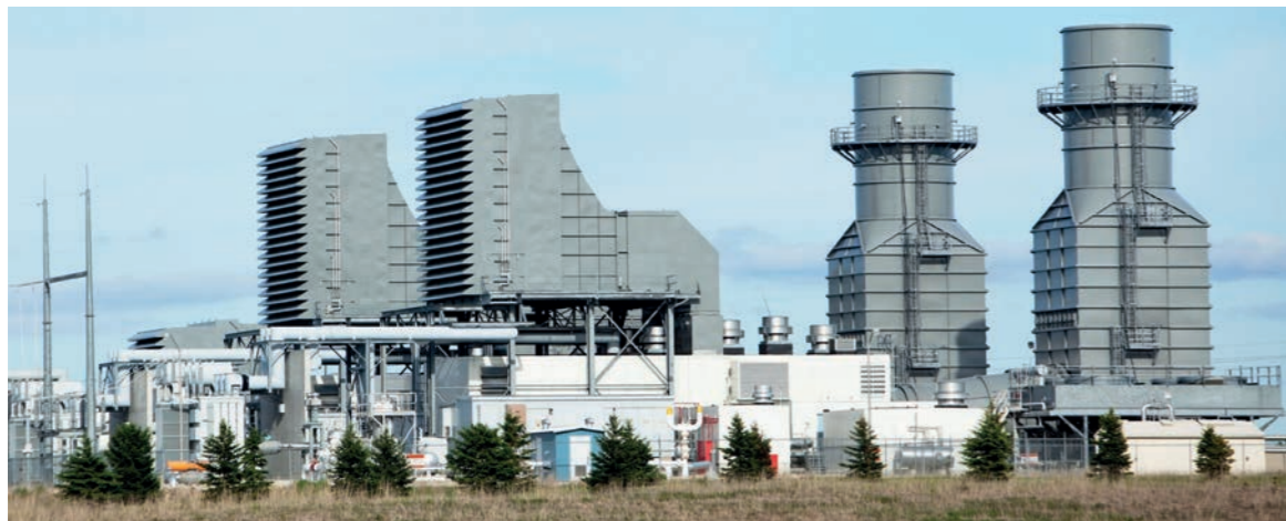
Figure 7: A gas turbine power station
