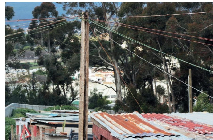
Figure 7: Illegal electricity connections in an informal settlement. Notice that there is no control box at the top of the pole for measuring electricity usage or for cutting off the electricity in case of a short circuit.
