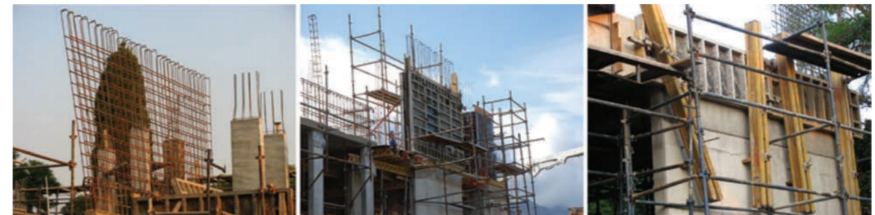
Figure 20: Steel reinforcement is placed inside a concrete wall of a big building.
