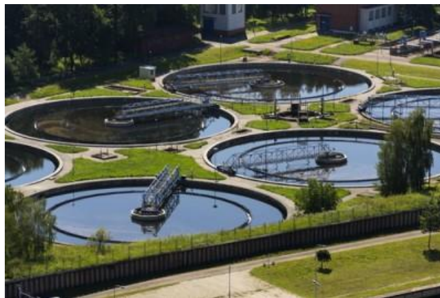
Fig 41. Aerial view of storage tanks in sewerage plant
