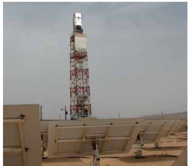
Figure 10: Mirrors in a solar-powered power station focus light onto heating towers.
