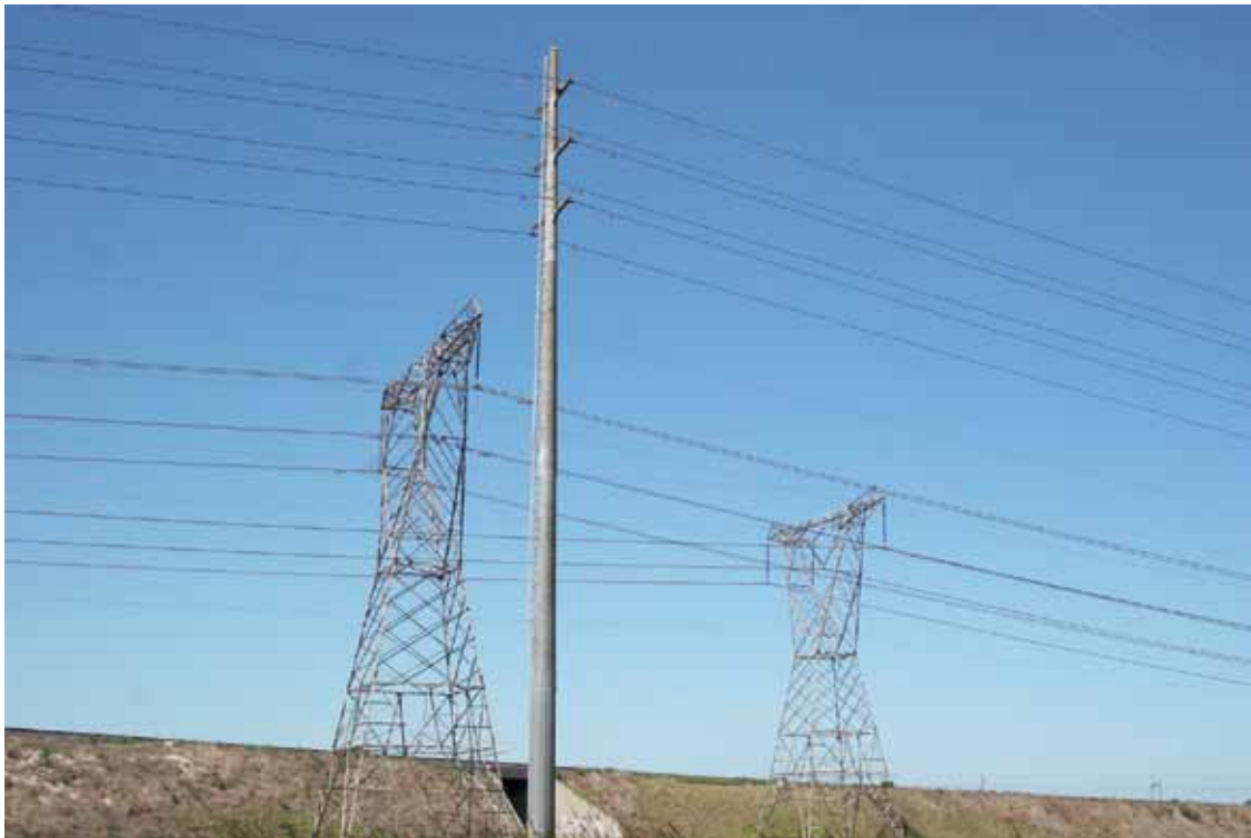
Figure 1: Pylons that carry the country's main electricity supply
