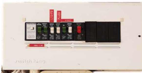
An electrical distribution board with circuit breakers
