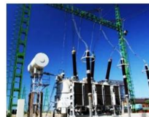
Figure 10 Transformers at substations reduce the amount of electricity. Electrical substations distribute electricity from power stations to homes, offices and schools
