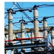
Figure 18 Power line with ceramic insulators
